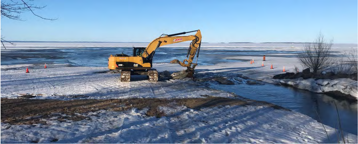
Figure 5 - Excavator at mouth of Parks Creek at Lake Nipissing, March 2022. Photo Credit P. Loranger.
