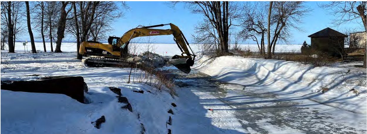
Figure 6 - Eva Wardlaw Conservation Area Parks Creek ice removal, March 2022. Photo Credit P. Loranger.
